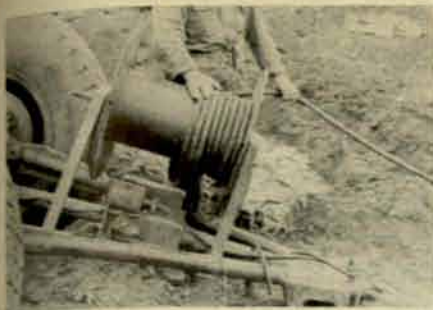
Cable rack in action.
